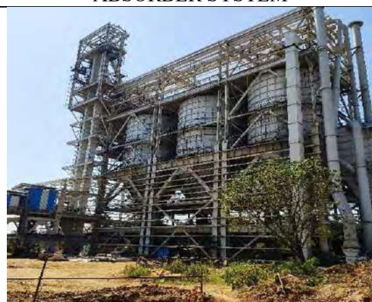
LIME HANDLING SYSTEM FOR BOTH UNITS
