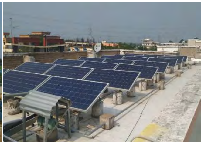
Roof top Solar
