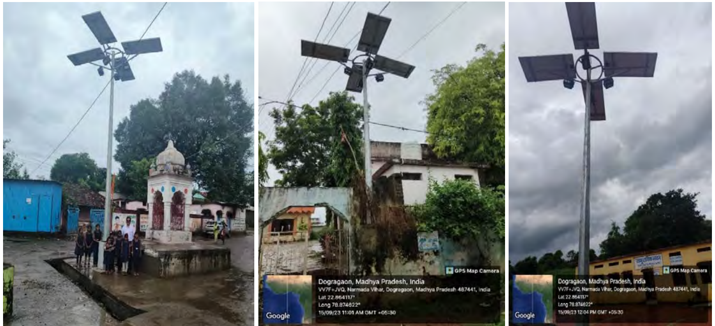
Solar High Mast Street Lights installed in Dongargaon, Gangai
