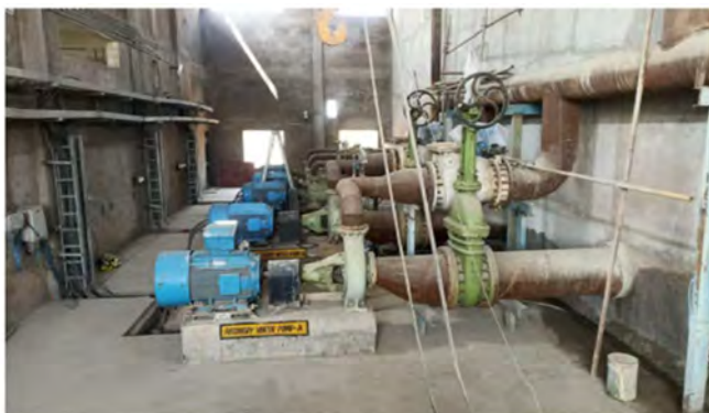
AWRS Pump House
