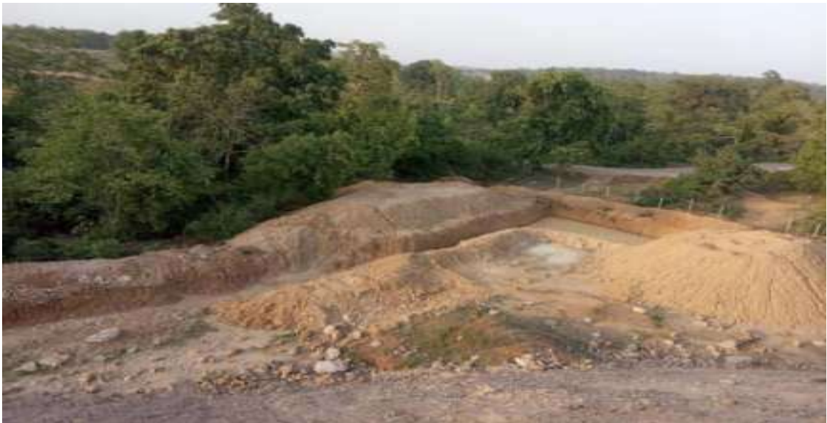
Garland Drain connected to settling pond
