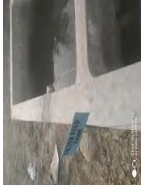
Filter Feed Tank
