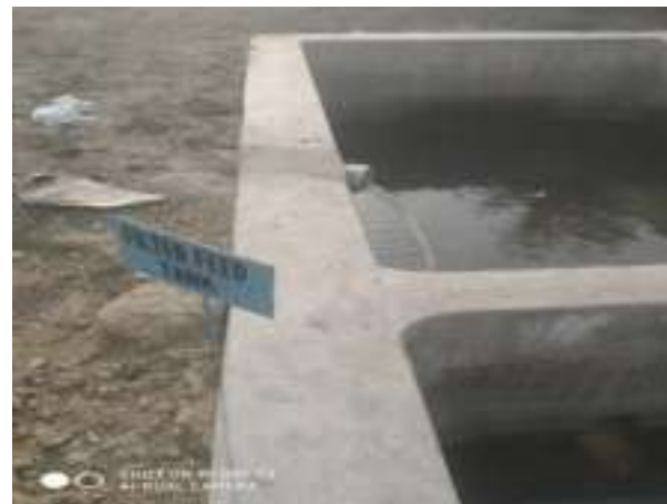
Filter Feed Tank
