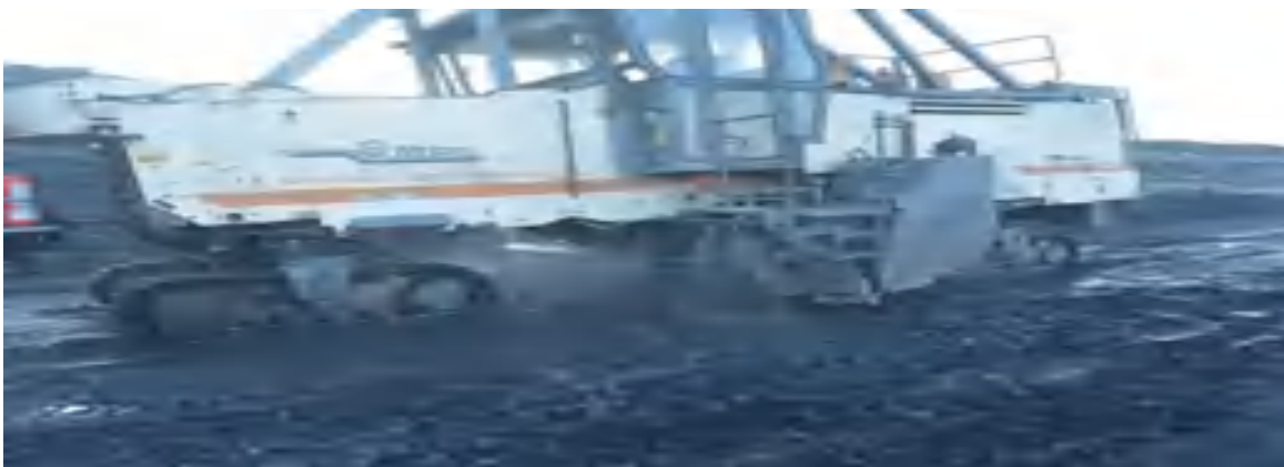
Interlocked Dust Suppression arrangement in Surface Miner
