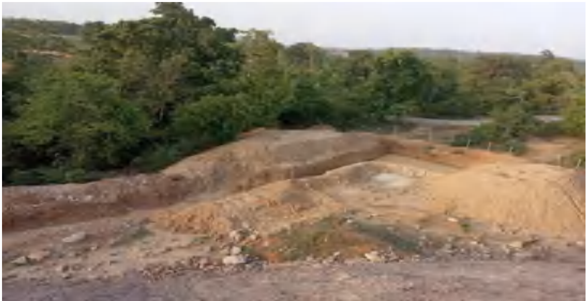
Garland Drain connected to settling pond
